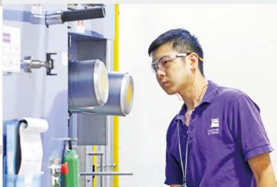
Clariant Plastics & Coatings (Taiwan) has advanced specialist spinning equipment, capable of meeting customers needs for a wide range of different product types (Photo courtesy of Clariant Plastics & Coatings (Taiwan) Co.,Ltd.)
