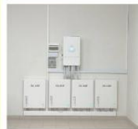
Residential Solar Projects
