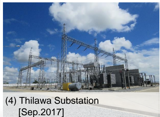
(4) Thilawa Substation [Sep.2017]
