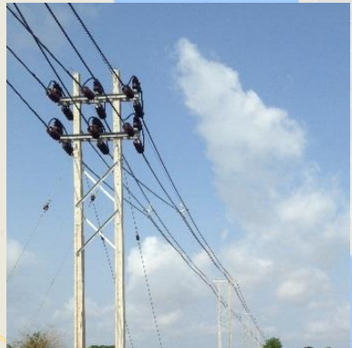
(1) 33kV Distribution Line Thanlyin S/S - SEZ [Apr.2015]
