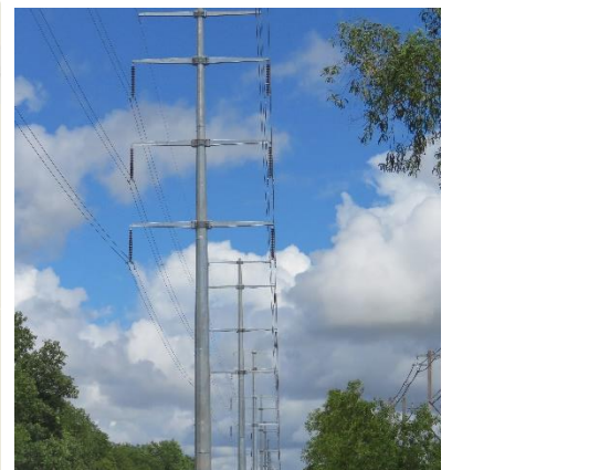
(5) 230kV Trans. Line [Nov.2017]
