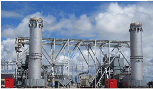
(3) 50MW Thilawa Power Plant [Mar.2016]
